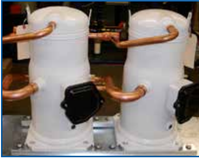
Typical refrigerant lines
